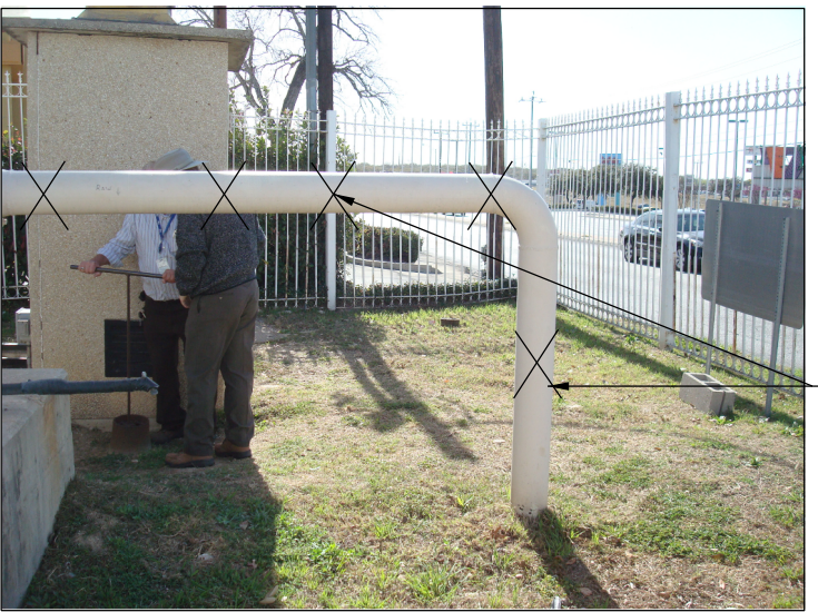
CUT AND CAP EXISTING 6" STEEL PIPE AND REMOVE ALL ABOVE GROUND PIPING. REFER TO EXISTING SITE PLAN THIS SHEET
